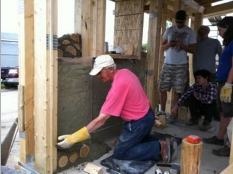
Cliff Shockey demonstrates how to erect a double wall to keep the cold Canadian air out of one's cordwood home.
